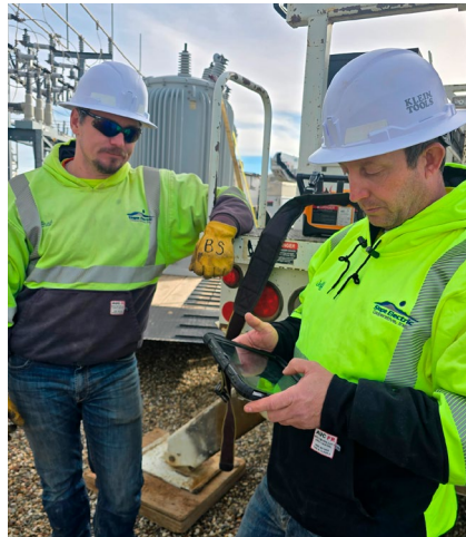
Journeyman lineworker Brad Schmitt and working outpost foreman Jeff Boynton , gather for a tailgate before starting a substation project.
