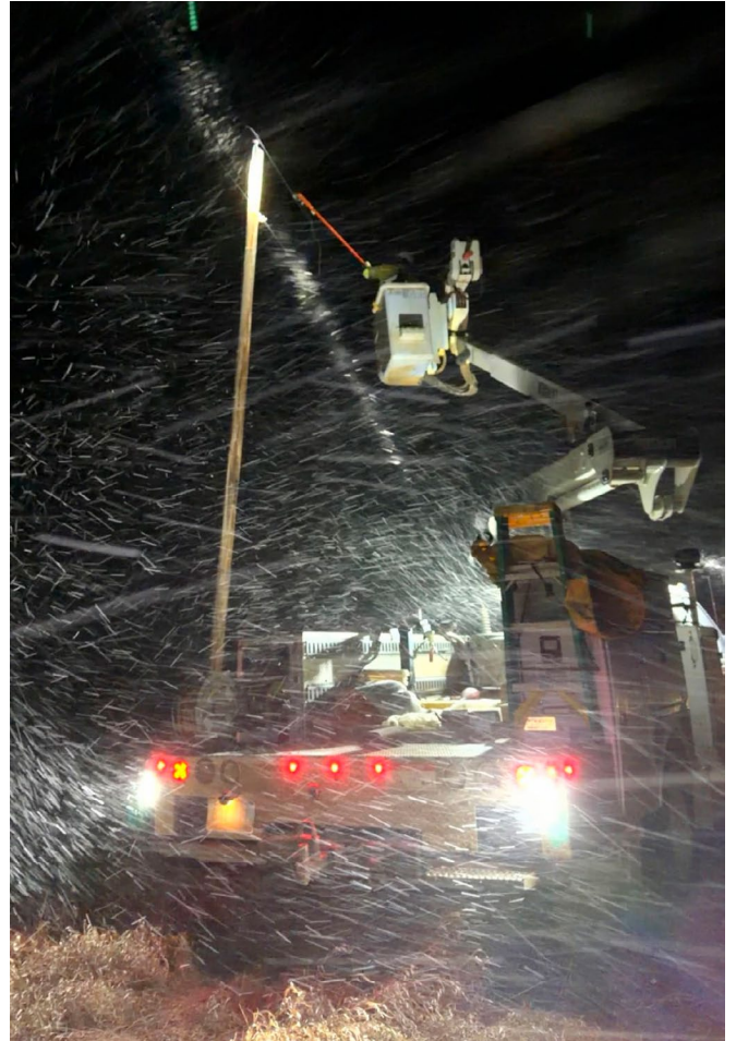
Cooperative employees are ready to respond to outages no matter the time or weather conditions.
